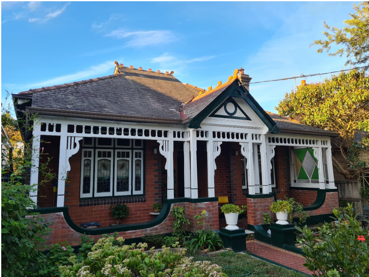
Image 1: Property in Euston Road, Hurlstone Park after painting works to front timber work funded by the previous heritage grant fund round.
